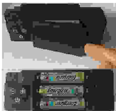
Batteries in the Gas Valve Controller Mounted at the front of the stove
